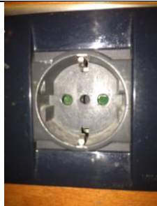
Electrical outlet in hotel rooms
