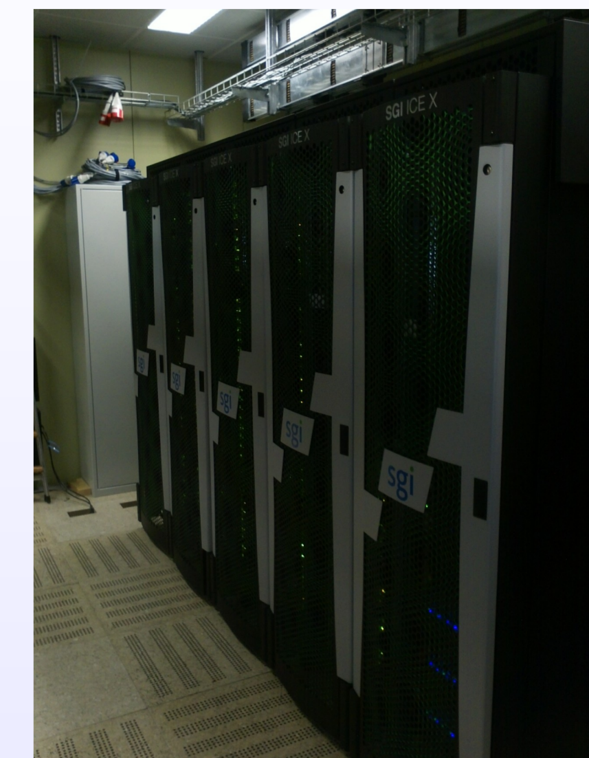
Figure 1: HPC system at ZAMG
