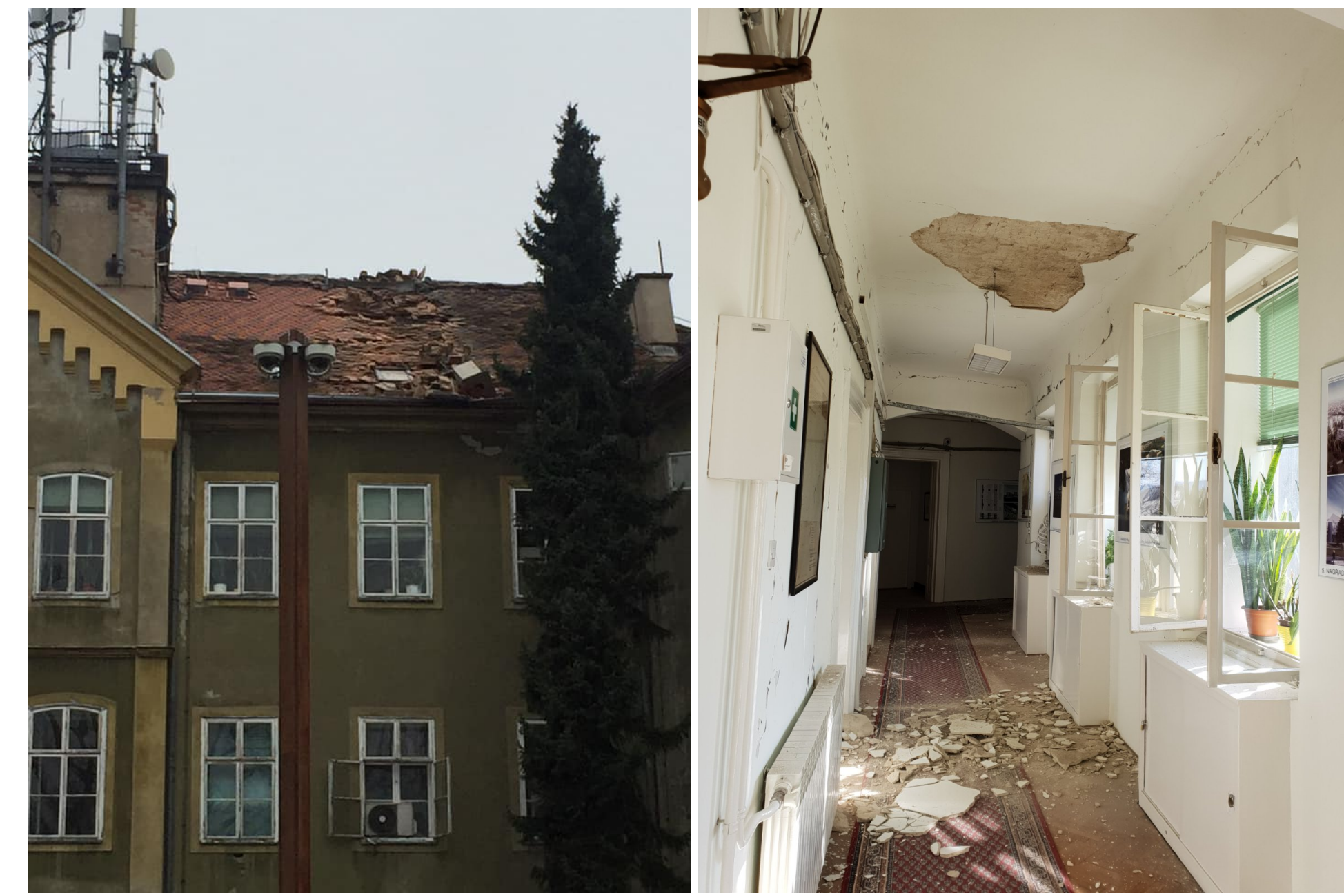
Figure 1. The impact of earthquake in Zagreb on DHMZ building
