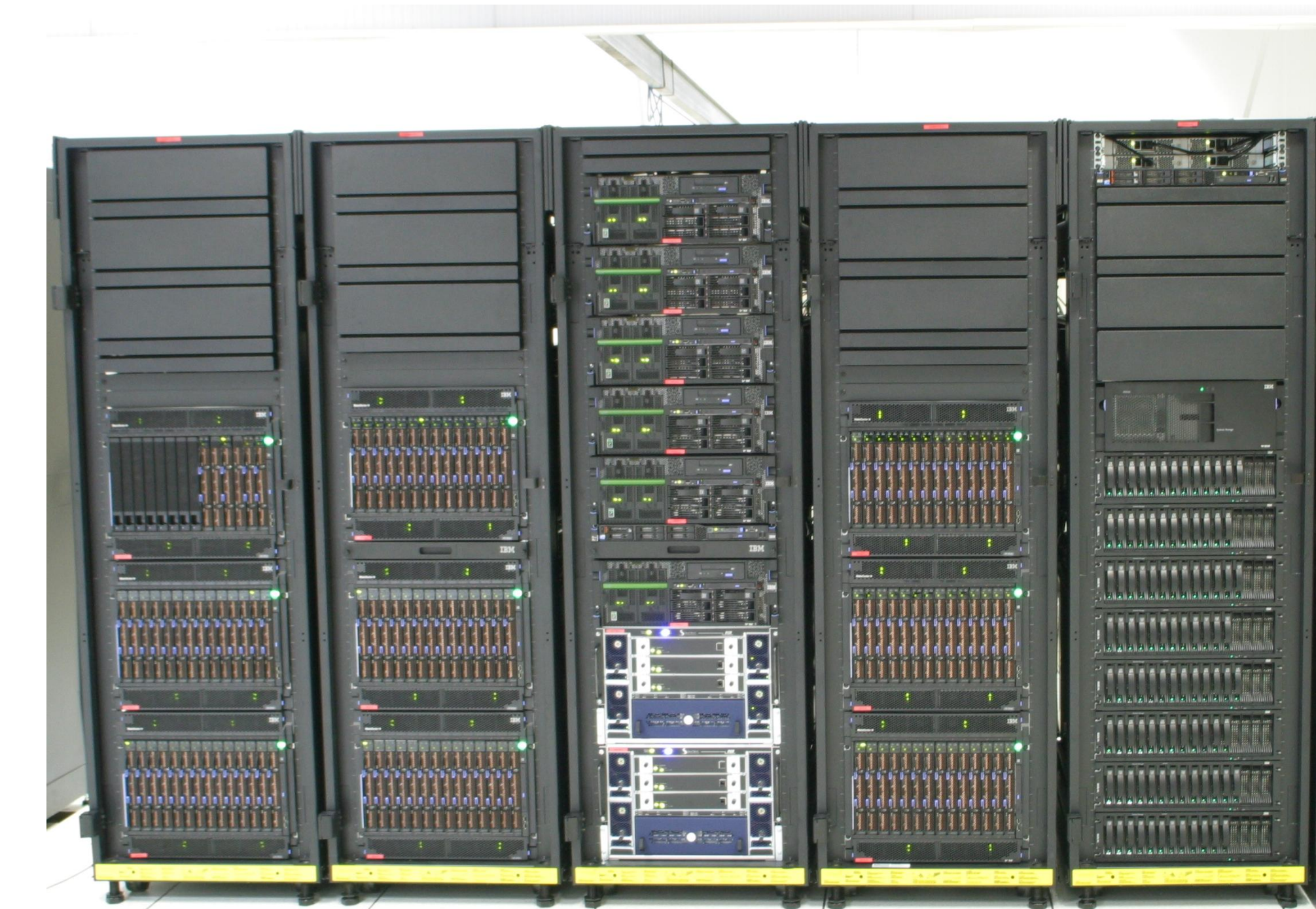
Fig 1 : IBM HPC (Power 6+, JS 23 & JS43, P520, IB Switch, DS5100, SAN Storage)
